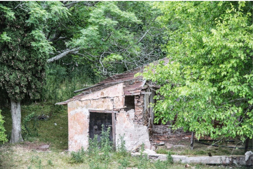
Photo 5. Old abandoned house.
